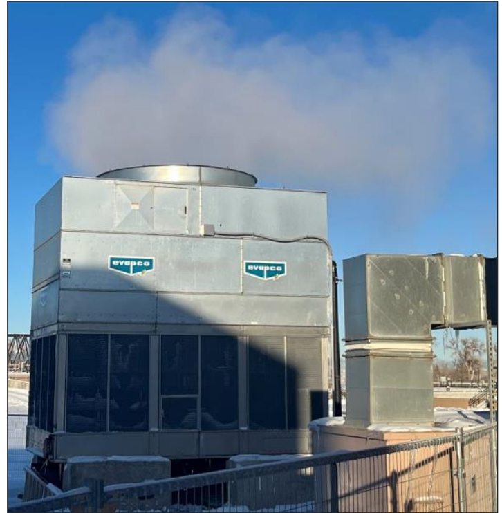
NTP effluent temperature demonstration cooling tower
