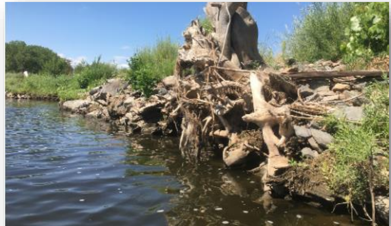
Anchored cottonwood root was providing bank stabilization and fish habitat at our Phase III Instream Habitat Improvement project along the South Platte River in Brighton, CO.
